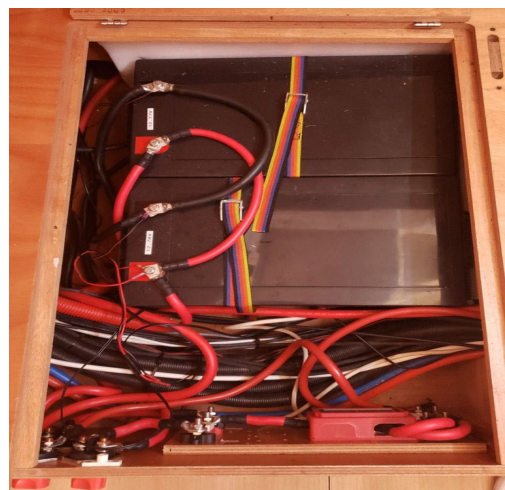
Fig. 16.8: ...and on the port side with many cables.
