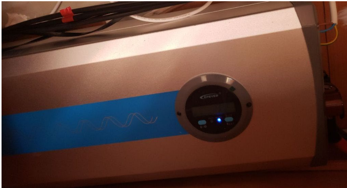
Fig. 16.15: The 3kW inverter for AC power supply.
