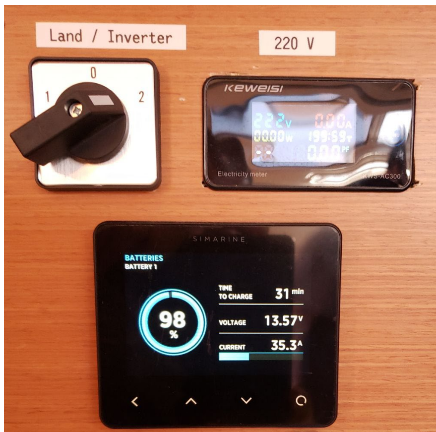
Fig. 16.16: Switch for shore power/inverter and measuring instruments for direct current (12V) and alternating current (220V).
