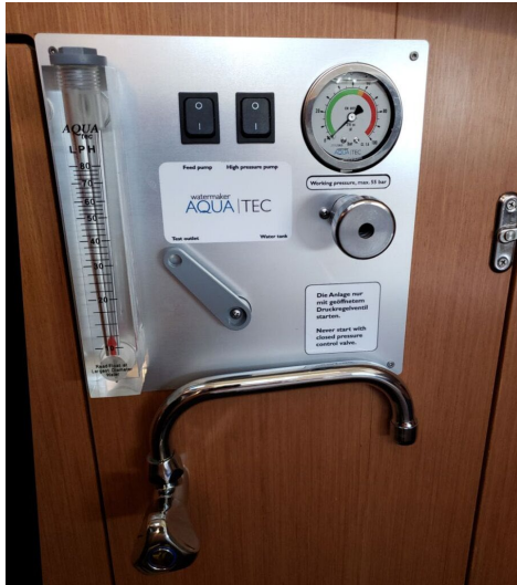
Fig. 26.26: The control panel of the water-maker.
