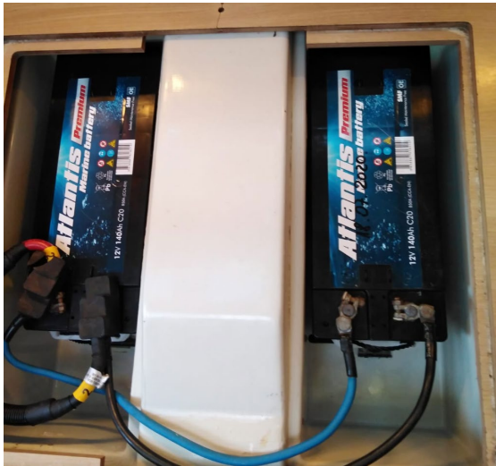
Fig. 8.8: Old battery bank (280Ah, lead-acid).
