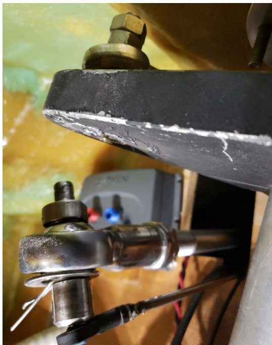
Fig. 28.4: The bolt that connects the autopilot's thrust arm to the rudder quadrant is broken. Fatigue fracture?
