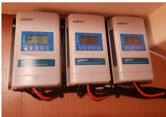
Fig. 16.13: The three solar charge controllers.
