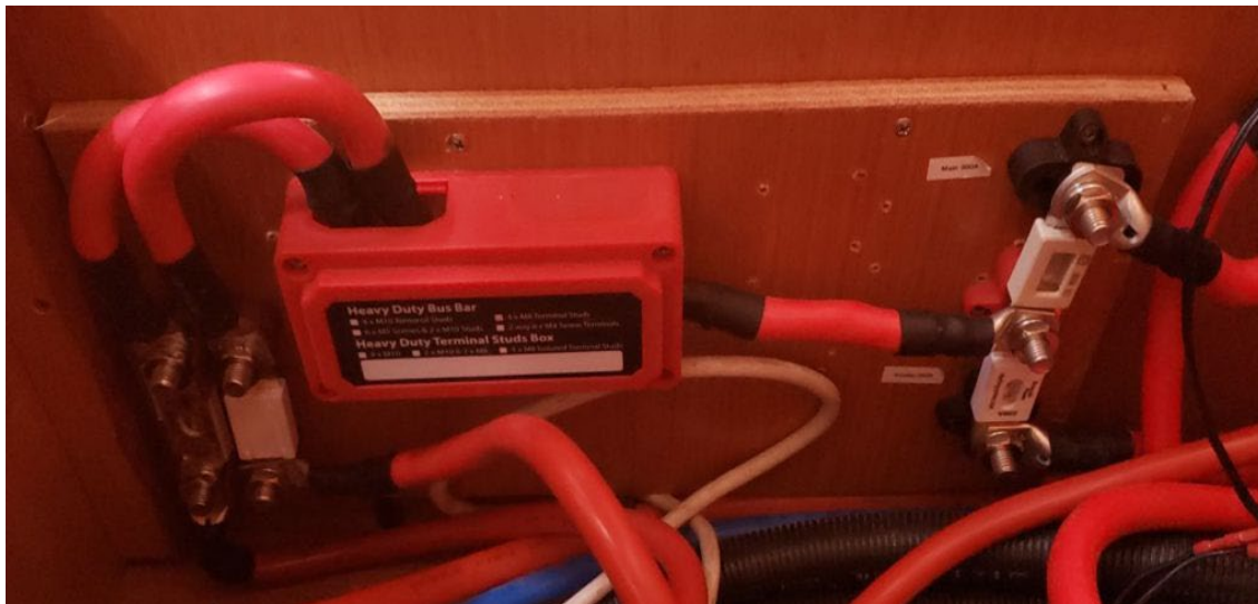
Fig. 16.10: The positive busbar with fuses.
