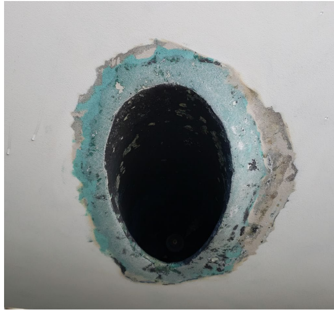
Fig. 26.17: The leaking inlet into the bow thruster tunnel.
