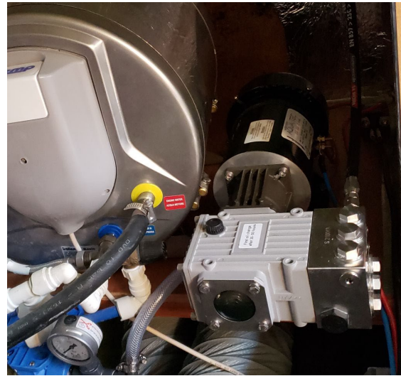
Fig. 26.27: The high-pressure pump next to the boiler.
