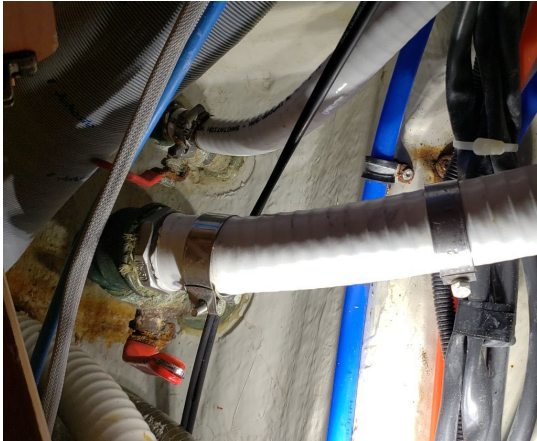
Fig. 26.13: Seacocks from the inside. Heavily corroded.
