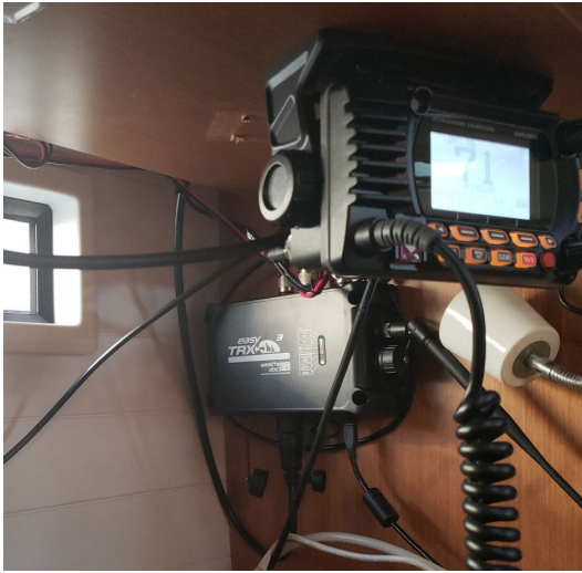
Fig. 8.10: AIS transceiver, quite inconspicuous in the corner.
